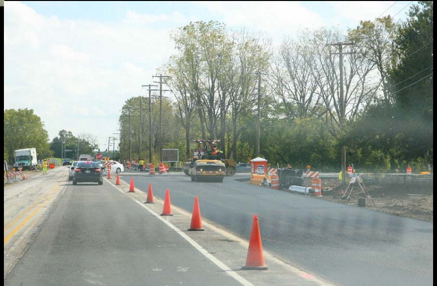
Crews place binder for pavement widening on the Huntley Rd at Galligan Rd Intersection Improvement
